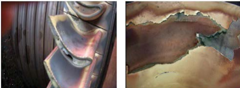
2, 3. Visual inspection of critical parts during disassembly revealed tip burning of first-stage buckets (left) and TBC loss from the DLN combustion liner (right)
